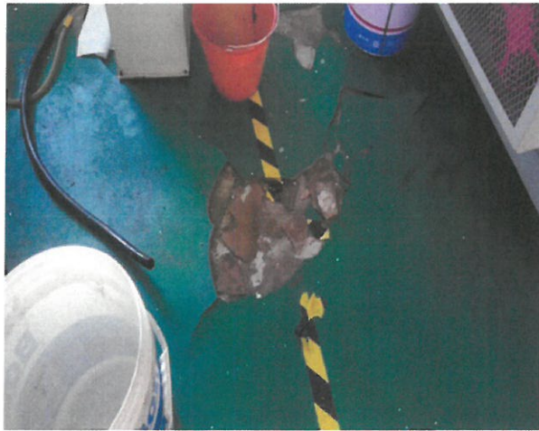
CNC工廠地板鋪面破損
